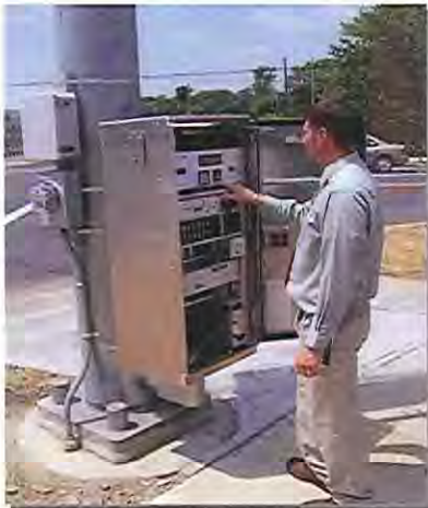
Type 2070 Traffic Controller Elmira, NY
